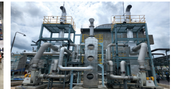
CTO - Air pollution prevention equipment
