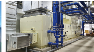
MW - Dehumidification equipment
