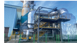
SCR - Air pollution prevention equipment
